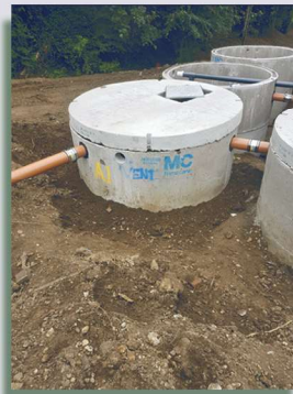
Concrete ring treatment plant
