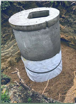
Borehole Drainage System
