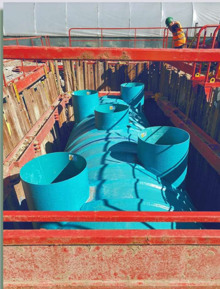
Commercial Treatment Plant
