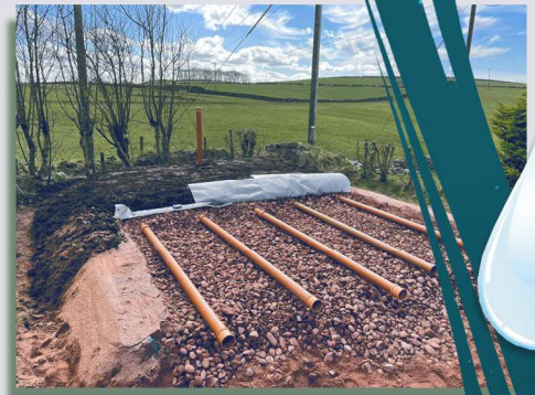
Drainage mound to BR478 plant
